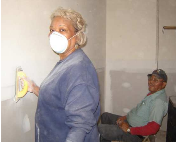
Pastor Gant rolled up her sleeves to help sand the new sheetrock. Ed King (background) cheered the Team on and gave direction daily.
