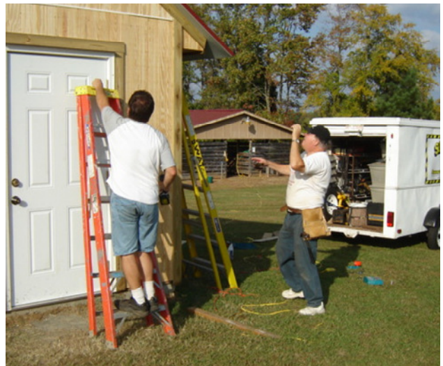
Installing siding and trim on the pump house. Doesn't it look great!
